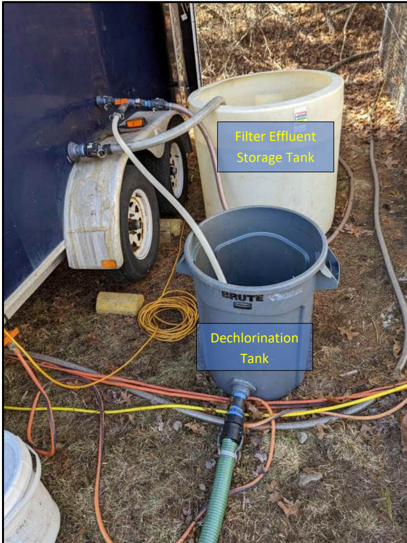
Figure 2.20: Pilot Effluent Tank and Waste Discharge
