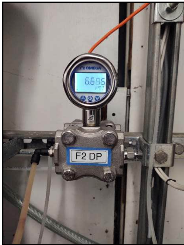
Figure 2.09: Differential Pressure Gauge for Filter F2 (typical of 3)
