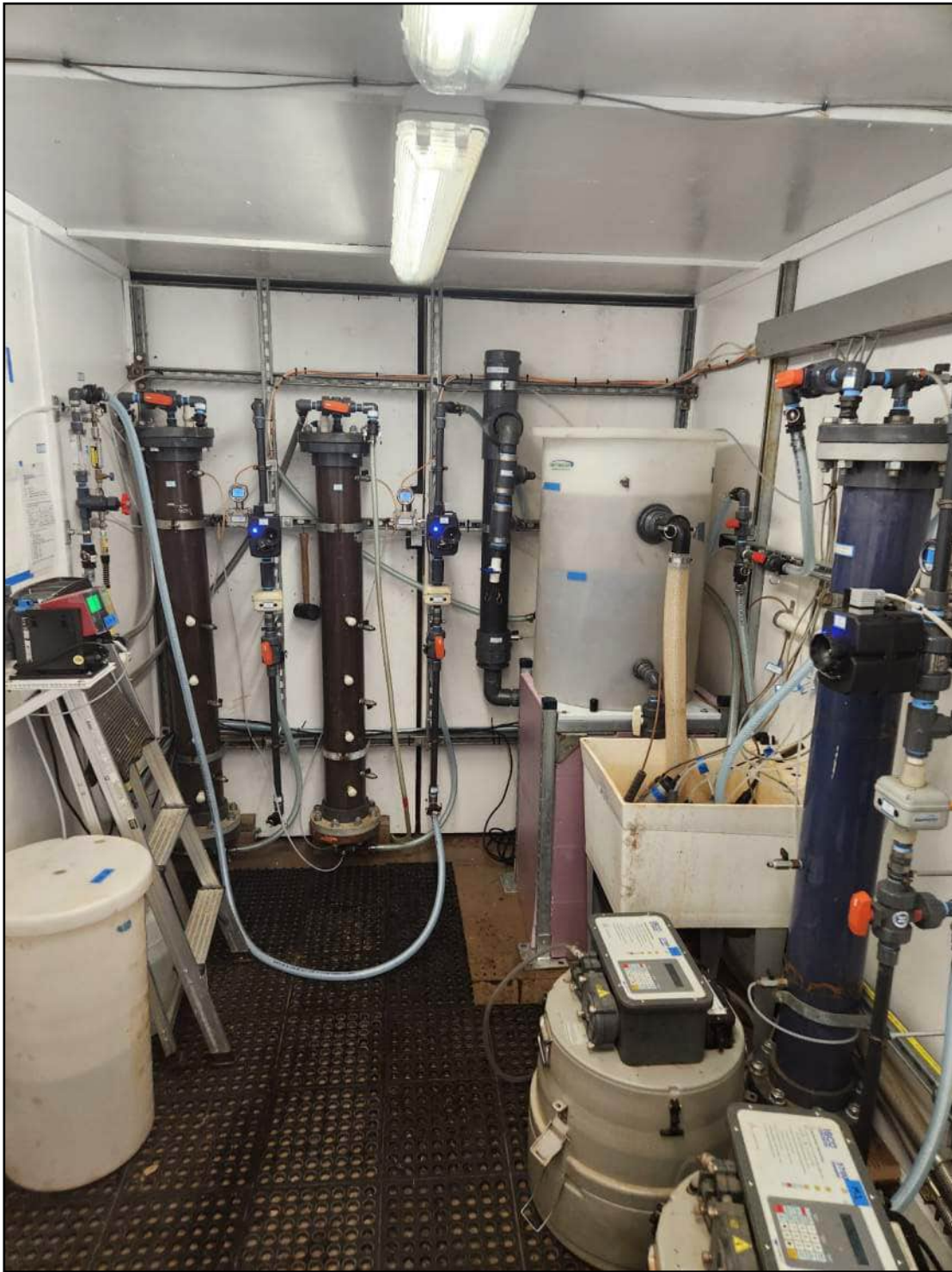
Figure 2.05: Interior of the Biological Pilot Trailer
