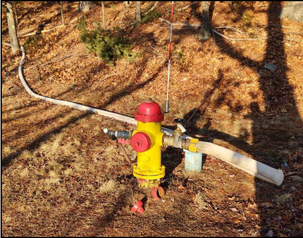
Figure 2.01: Pilot Connection at Wellfield 2 Raw Water Hydrant
