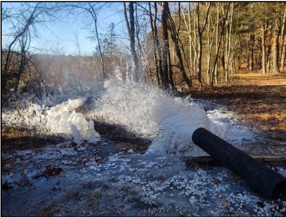
Figure 2.02: Raw Water Discharged to Waste
