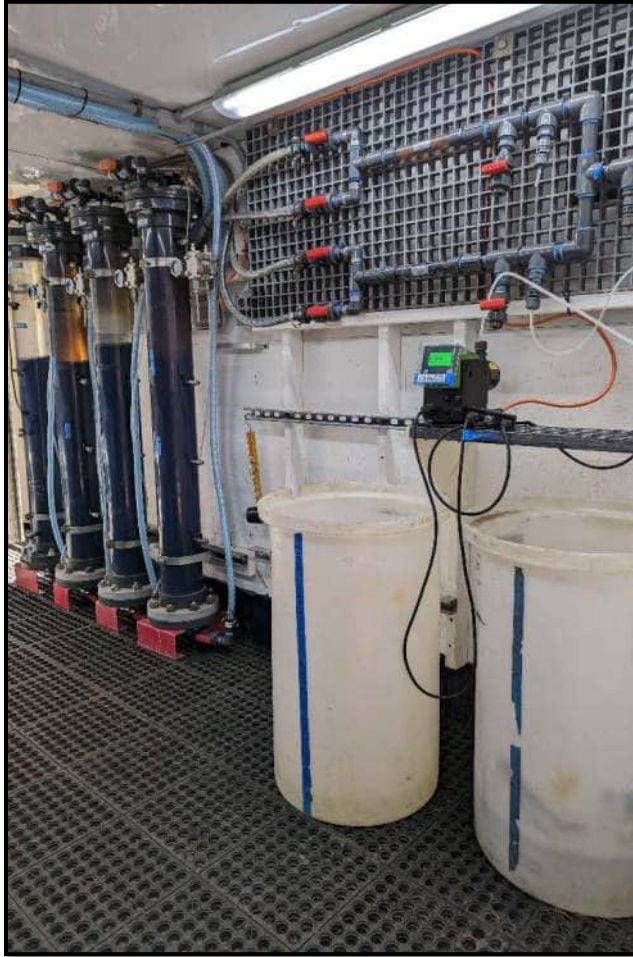
Figure 2.16: Sodium Hypochlorite Feed Pump
