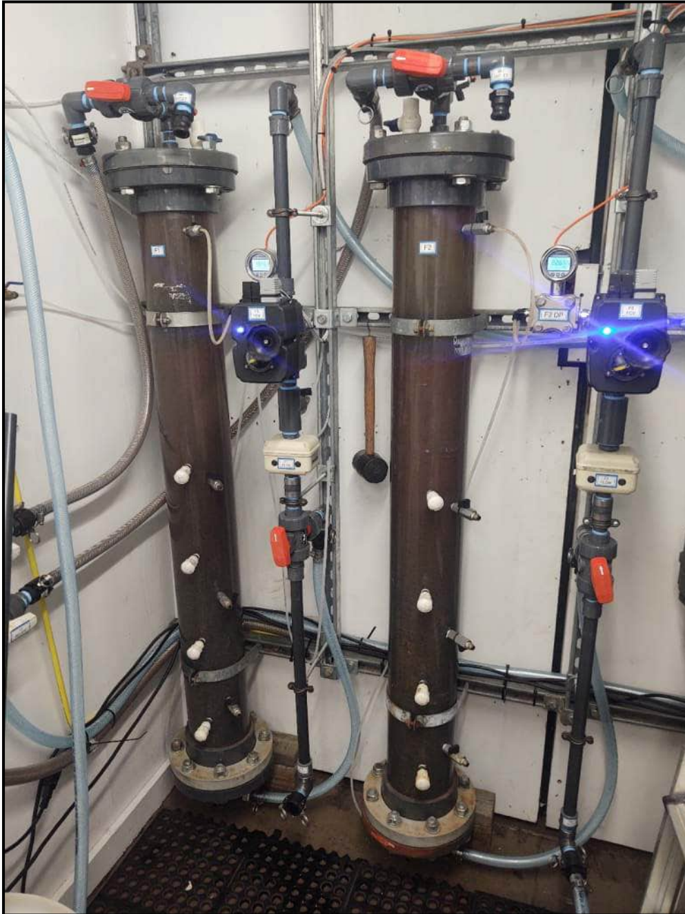
Figure 2.08: Filter Vessels F1 (left) and F2 (right)
