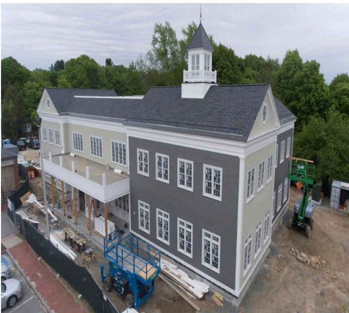
New Town Hall rendering (above) and New Town Hall under construction (below; photo June 2019). Source: https://www.townofsharon.net/home/pages/new-town-hall-project
