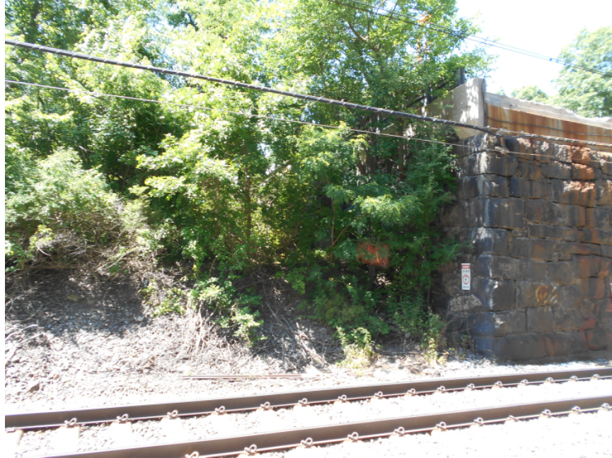
Photo 7 – Southwest retaining wall at the west abutment from the east side of the MBTA tracks. Grades slope upwards to Maskwonicut Street. Thick vegetation is present.
