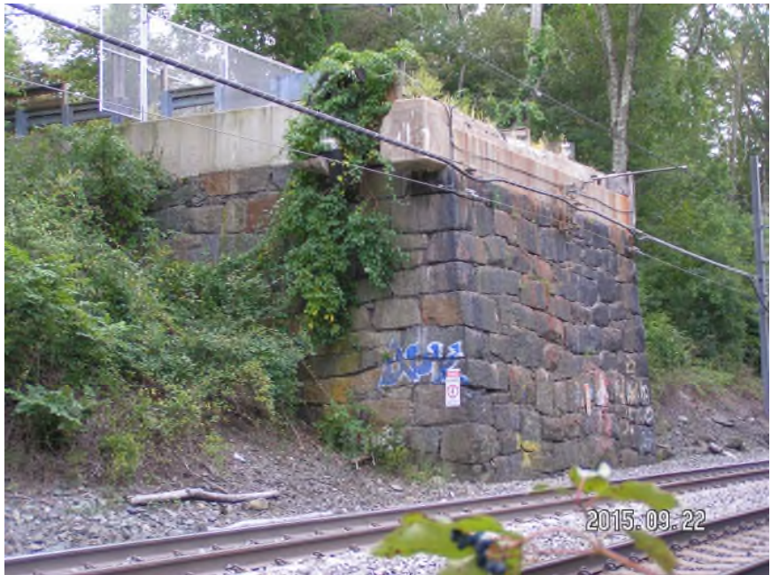
Photo 4 – The east abutment and northeast retaining wall from the railroad tracks looking southeast.
