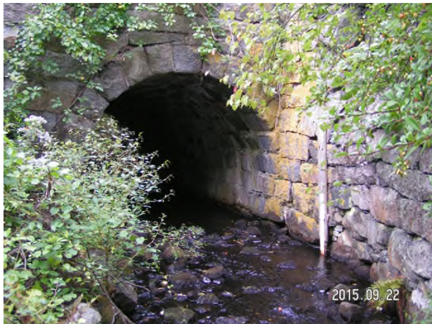
Photo 6 – Beaver Brook and the stone arch culvert beneath the west end of the retaining walls at the west abutment. The retaining walls extend along the brook upstream and downstream of the roadway.
