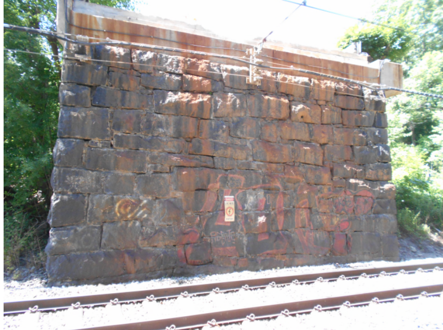
Photo 5 – The face of the west abutment from track level. Overhead railroad wires are supported from a bracket mounted directly to the abutment.
