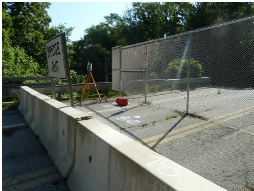
Photo 2 – Jersey barriers and security fence at the west approach. Note the timber covered metal guard rails.
